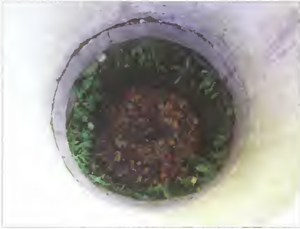
Figure 2.38. The interior of the spring well showing the existing water level (leaf-covered) and lower fern-lined stone walls that predate the courtyard. The upper limestone section was added in c.1933. (Roger Williams National Memorial, 2009.)
